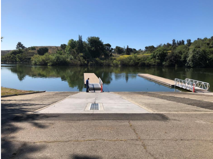
New cable-guided boarding float, cable housing, concrete landing, and gangways
